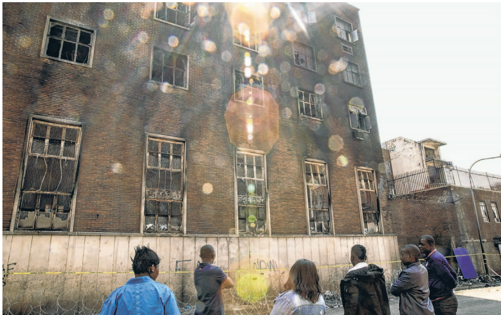
Onlookers outside the gutted remains of 80 Albert St. in downtown Johannesburg. At least 77 people died in the fire there early last Thursday morning.
