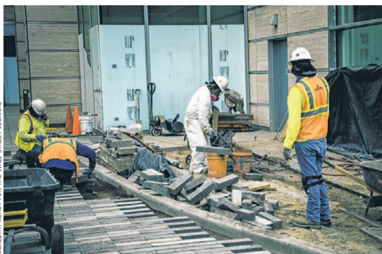
Work on what will be offices at Exxon Mobil headquarters in Texas.
