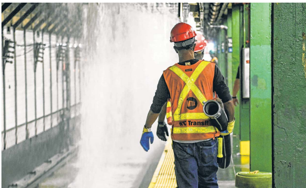
RAIN DELAY: A break in a 127-year-old water main under New York's Times Square sent water into the subway station on Tuesday.
