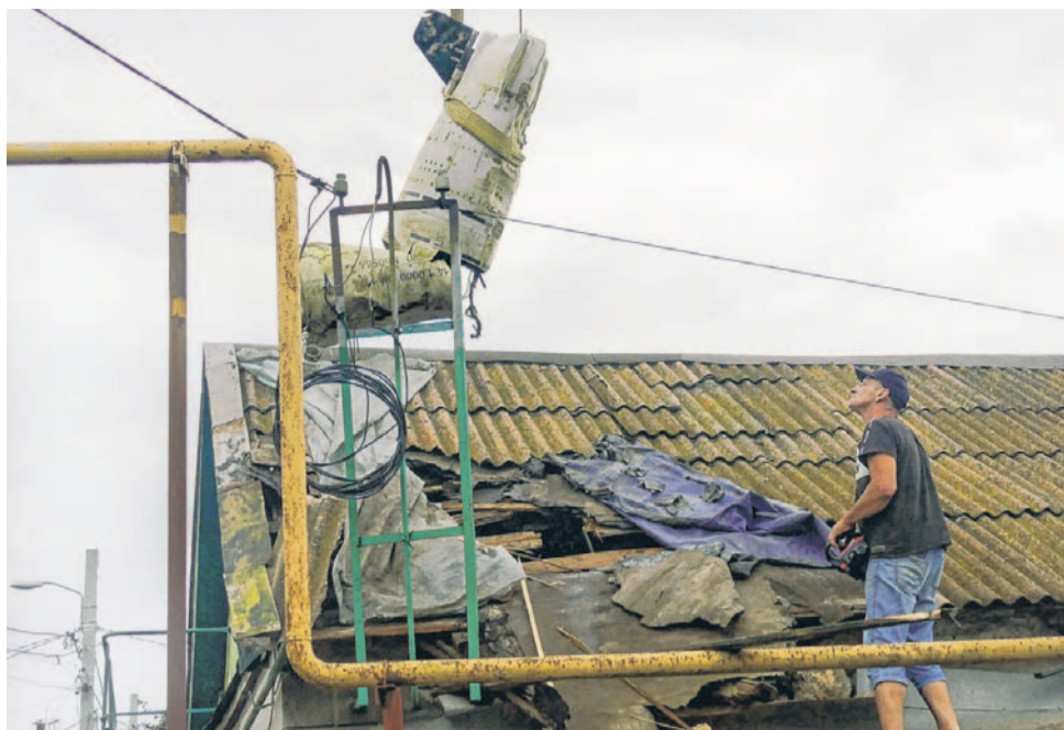
Workers remove part of a rocket through a hole in a building roof after an attack on Odesa.
