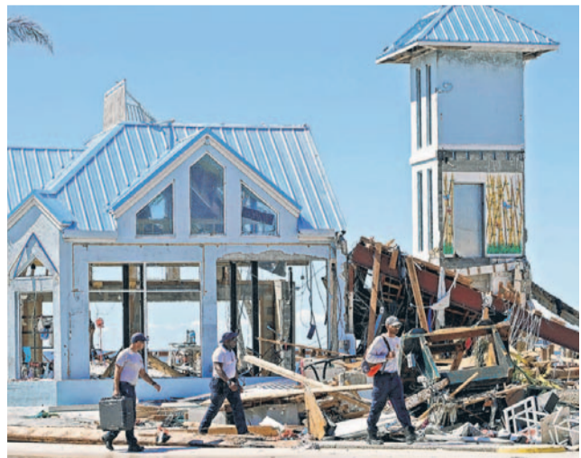
Damage in Florida from Hurricane Ian last September
