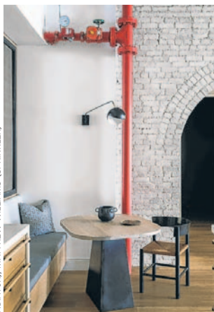
FRIENDLY FIRE Red makes this Tribeca loft's sprinkler a modern design feature.
