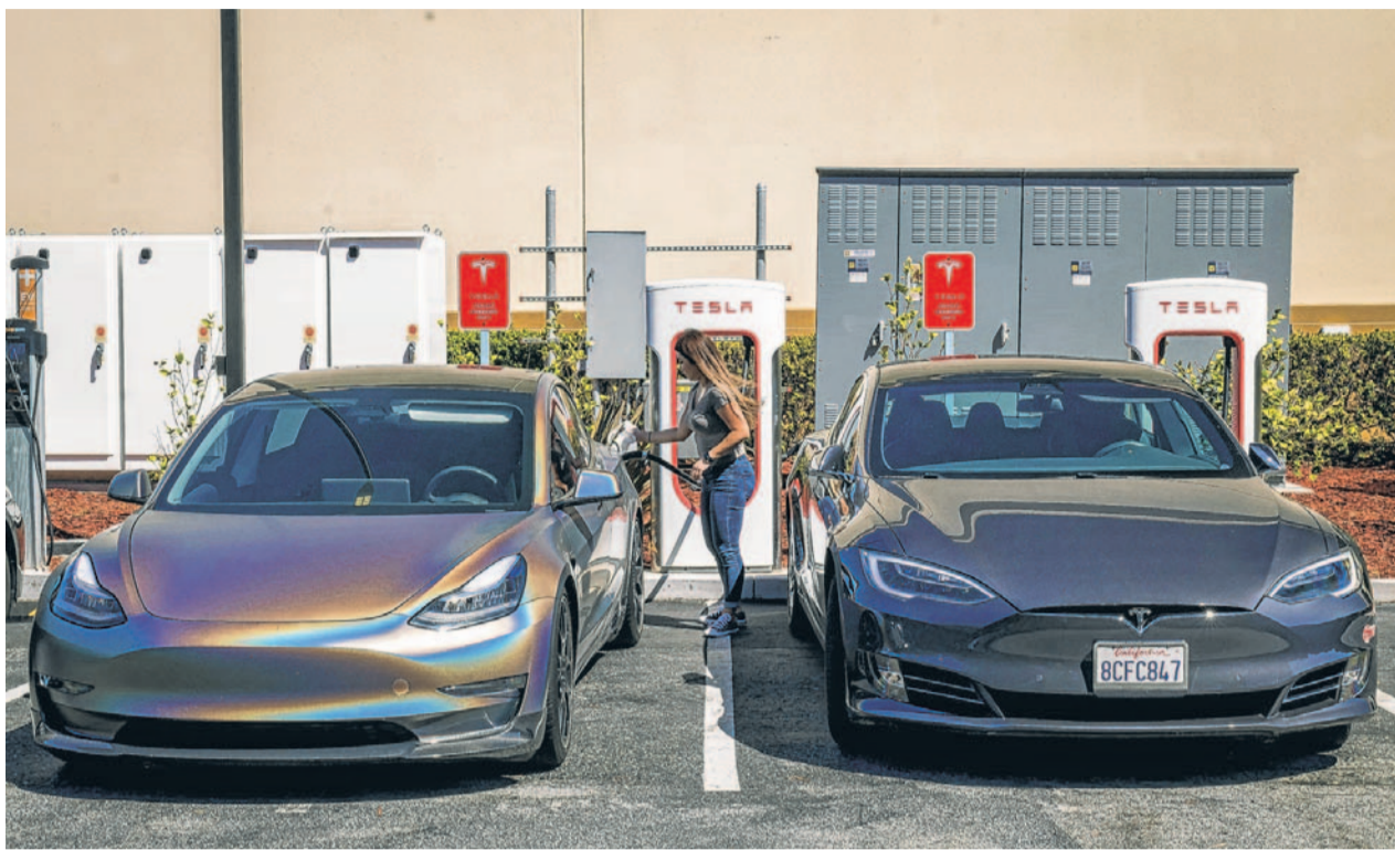
Owners of EVs from Ford and General Motors will gain access to 12,000 of Tesla's approximately 17,000 Superchargers.
