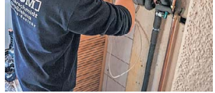
Installation: a plumber fits a gas boiler in Saxony ahead of the ban
