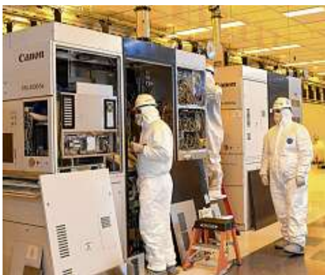
Workers attend to equipment in the clean room at a Wolfspeed silicon-carbide fabrication facility in Marcy, N.Y.
