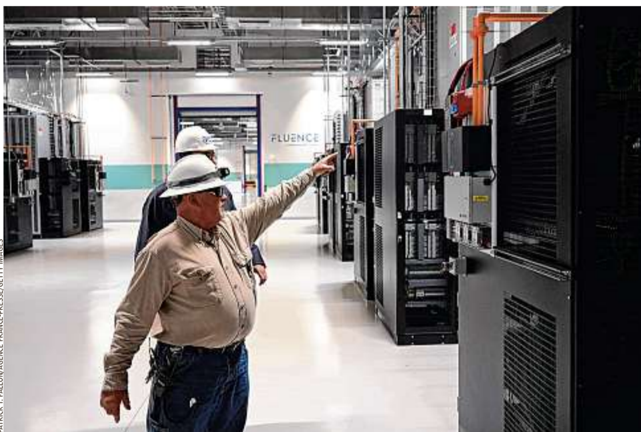
Battery storage is especially important in states like California, which rely in part on solar power that can't be generated at night.
