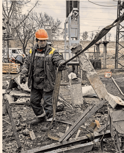
More than 40 per cent of Ukraine's energy infrastructure has been damaged, but engineers have had some success in shunting power around disabled parts of the grid. Ed Ramo/Getty Images
