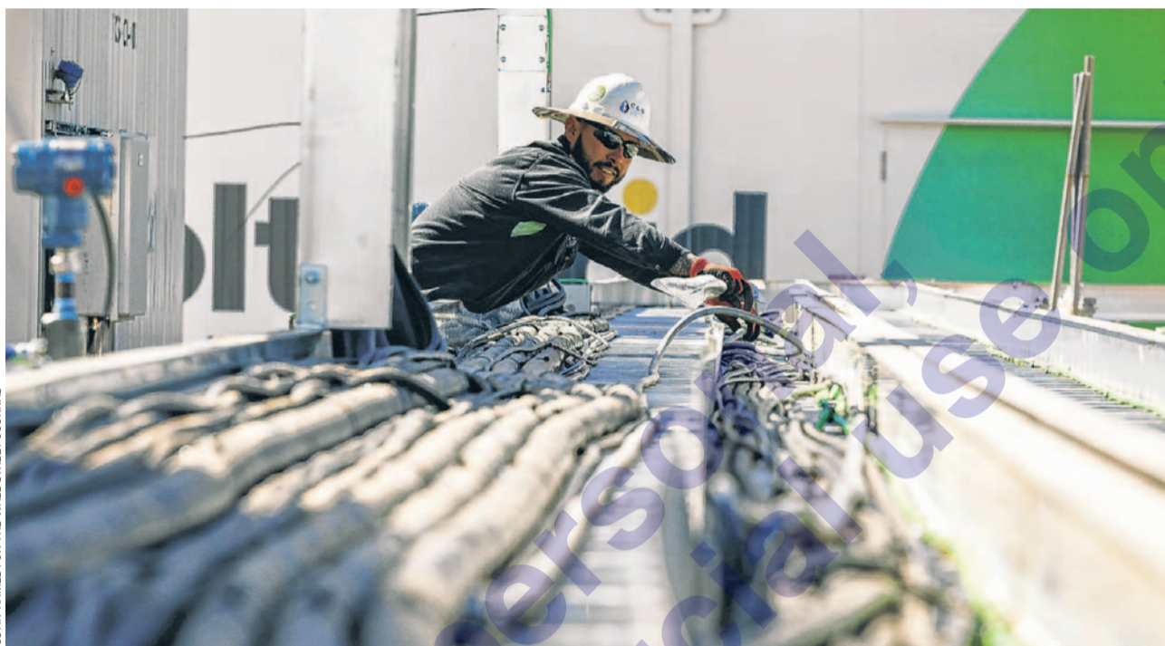
A compressor station feeds gas to pumps where it can be taken away for use elsewhere in Diamondback's Permian operation.
