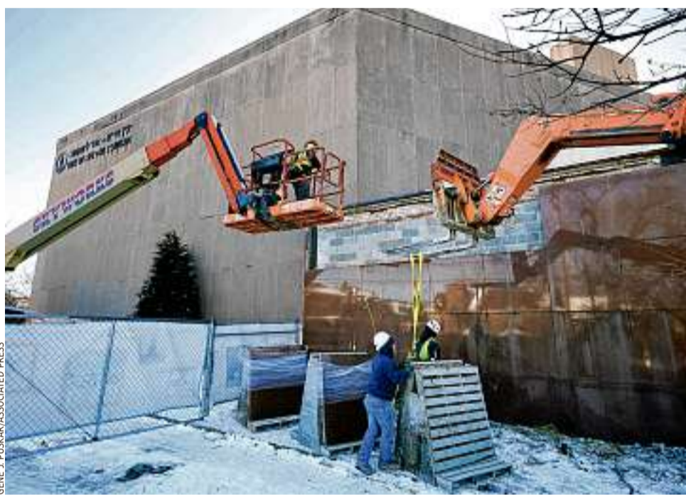
SOLEMN TASK: Workers begin demolition Wednesday at the Tree of Life building in Pittsburgh, the site of the deadliest antisemitic attack in U.S. history. Most of the structure will be removed and a new building constructed in a way that honors the 11 people killed there in 2018.
