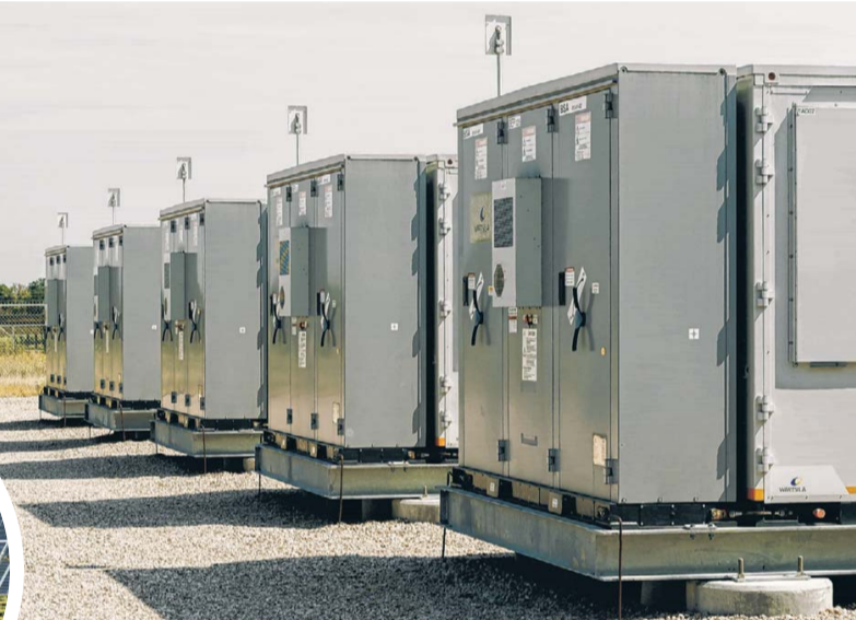
Battery storage at an Enel solar facility in Texas this month. In the state, which logged 10 demand records this summer, batteries helped avoid rolling blackouts one recent evening.
