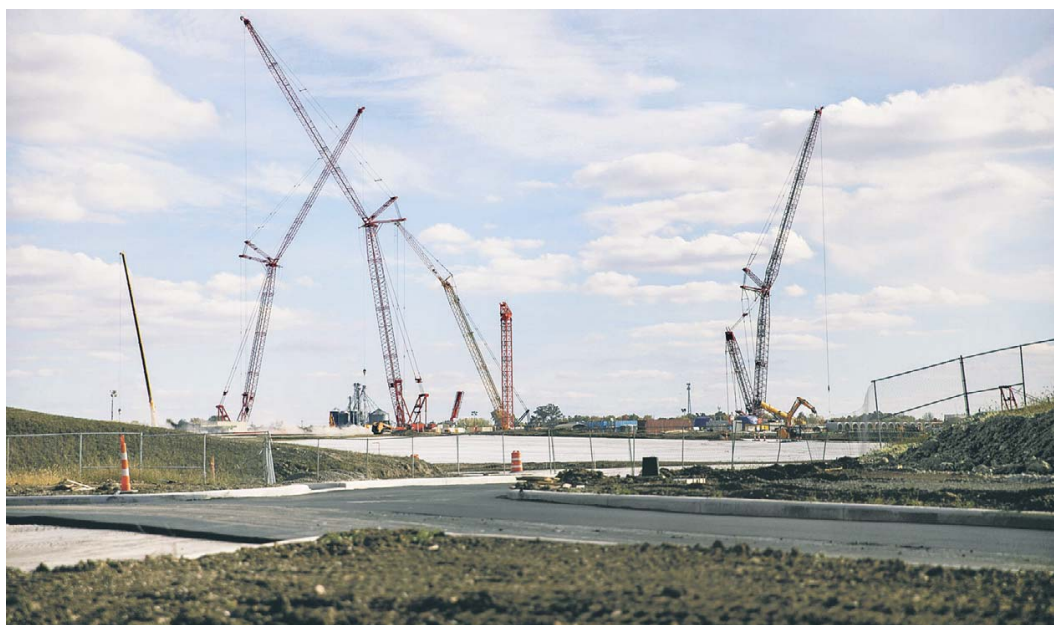
Above, construction at an Intel site in Ohio's Licking County in October. Middle, attendees at a Honda recruiting event at Columbus State Community College that month. Bottom, a student at the school uses a VR headset at a recruiting event.
